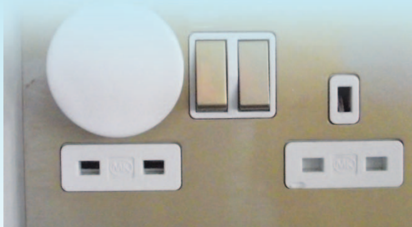
Figure 1 - Wrongly inserted socket protector.
