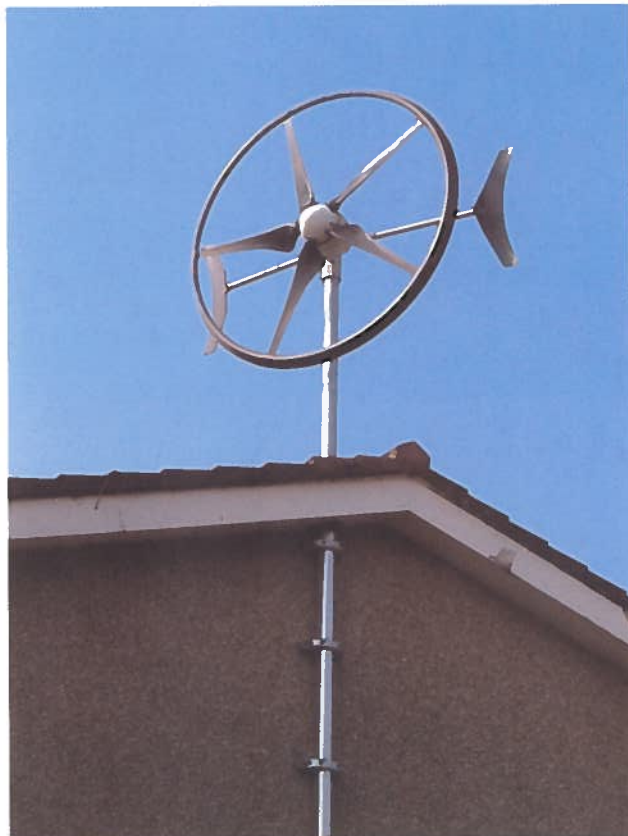
Figure 7 - School turbine installed at Collydean Primary
