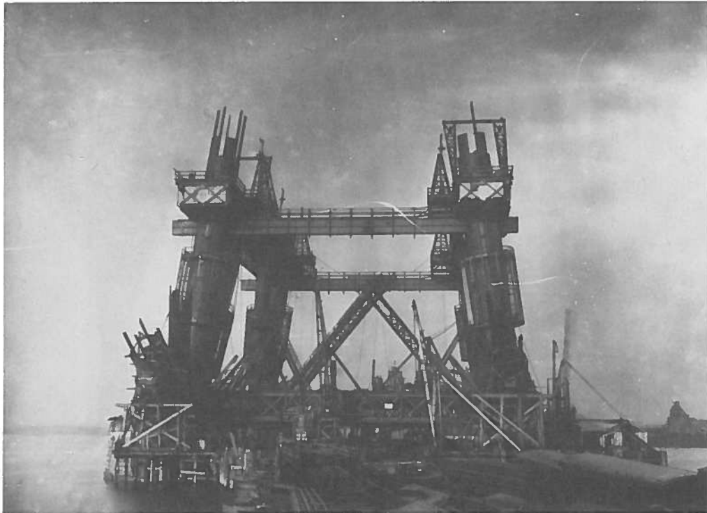
Figure 6 Forth Rail Bridge, the part built Queensferry cantilever in December 1886. Note the rivetting cages. (RCAHMS)
