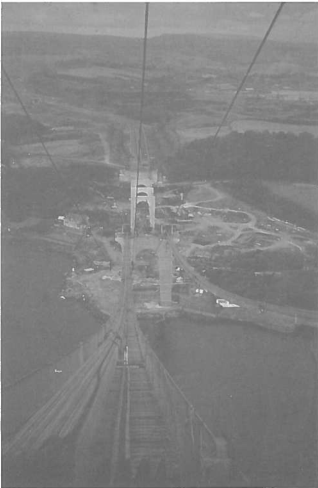
Figure 1 Forth Road Bridge. From atop the south main tower looking north to Fife. Taken during the fabrication of the main suspension cables. Unusually for the time, the tower construction used high tensile steel.
