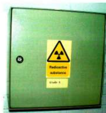
Figure 1 Radioactive sources cabinet
